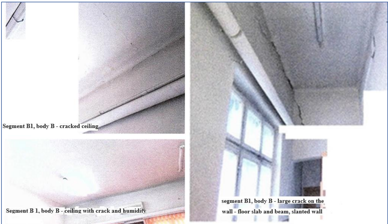
Fig. 6 – Damages of the inside elements
