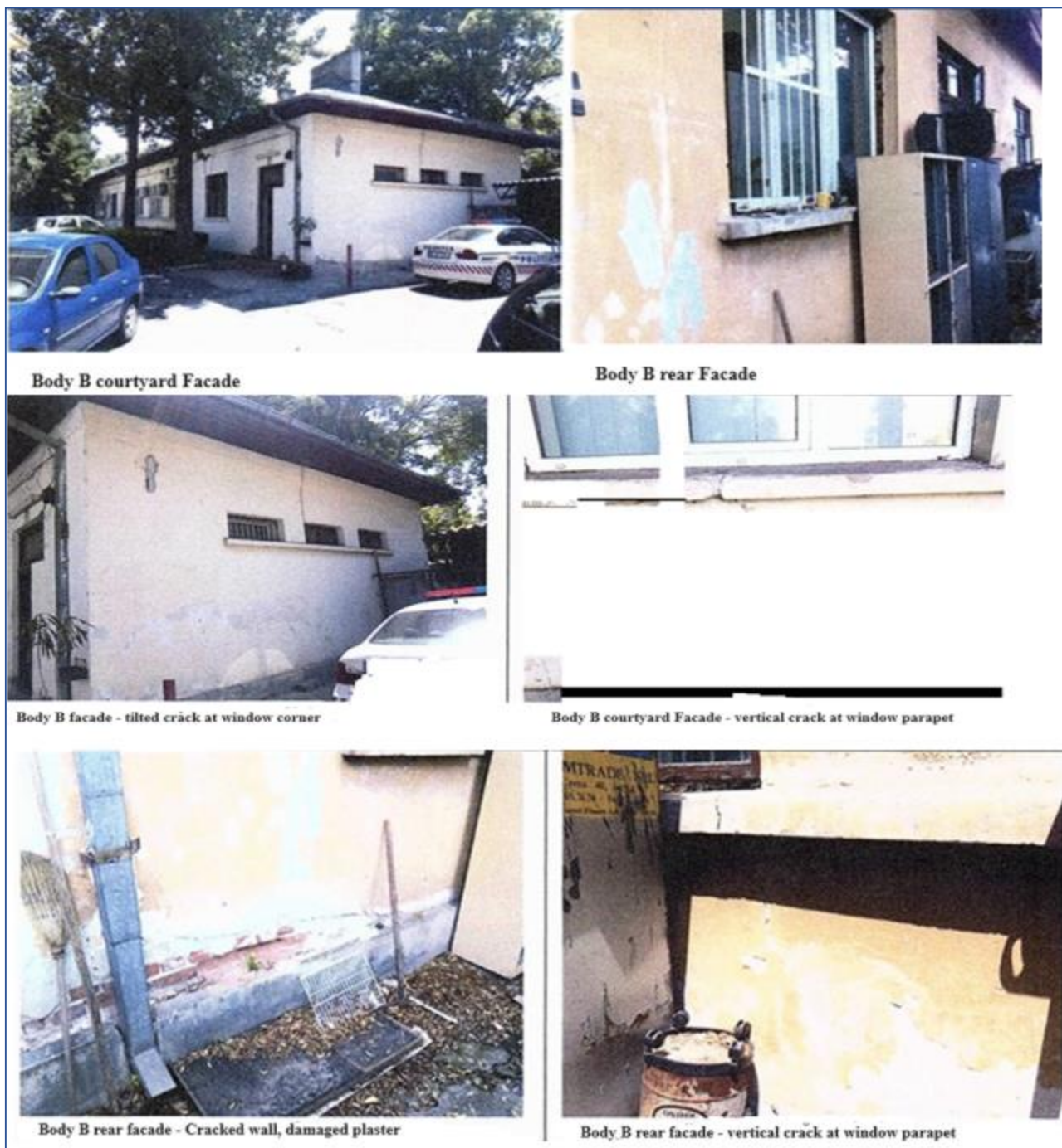
Fig. 4 – Body B facades damages
